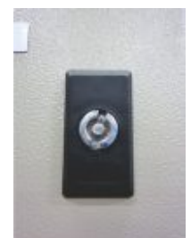
Access to the low voltage compartment can be restricted with the key-lock
