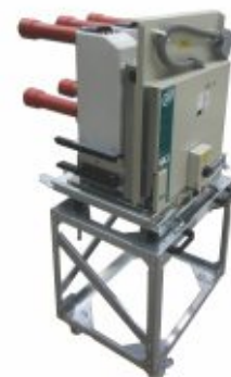
DOU is in the removed position
