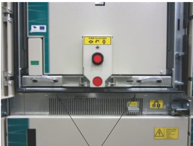
Openings for trolley guides
