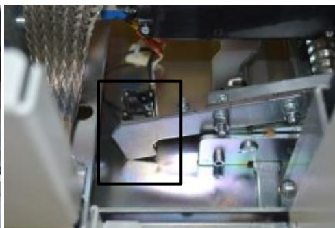
Position of not activated interlock inside DOU (voltage applied)
