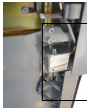
Earthing switch electromagnetic interlock
